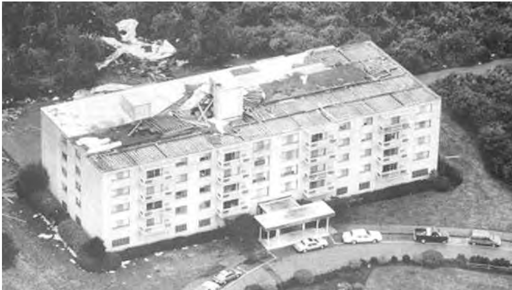
Figure 3-22. The destruction of the roof at the Admiralty Apartment building from the wind gusts during Hurricane Bob.
