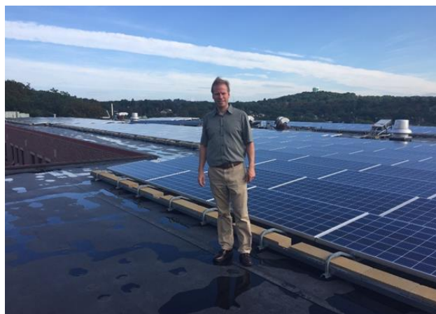
Solar array, Ottoson Middle School
